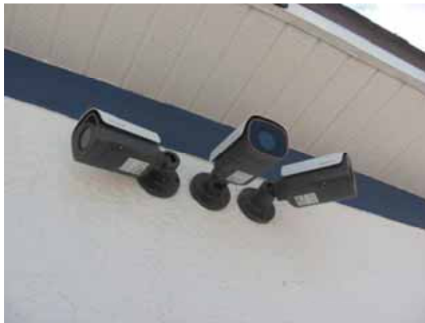
Security system cameras
