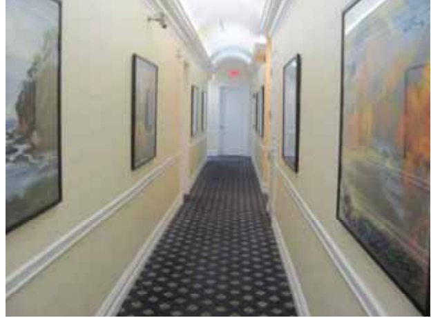
Paint finishes at the hallway
