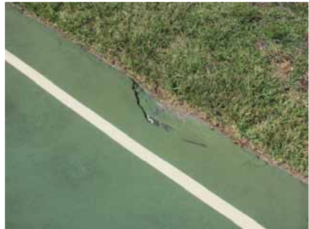
Basketball court – Note edge crack
